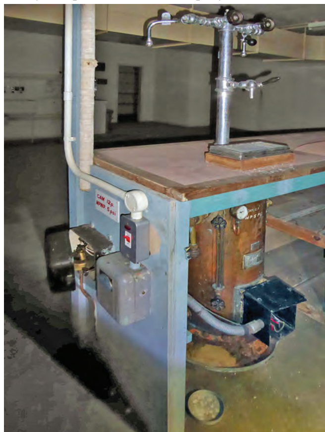
Kitchen boiler with pressure gauges and hot water outlet
